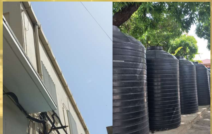
Gutters installed on the building direct water to a filtration system, which then transfers it to storage tanks.
